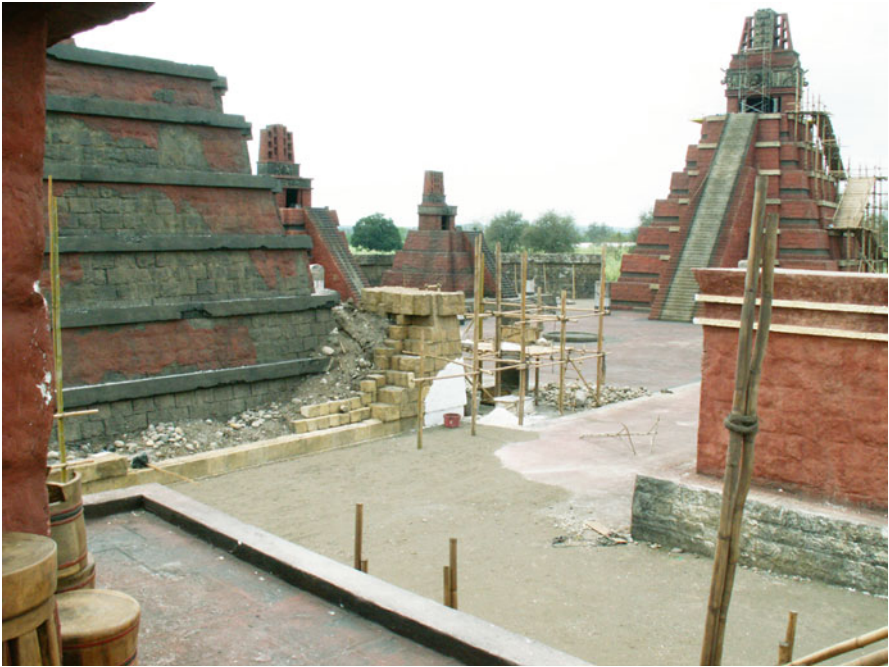
Fig. 8.20 The Central Plaza of the Apocalypso cityscape. Not the remodeling and construction underway on the weathered building on the left (Photo: R.D. Hansen)
