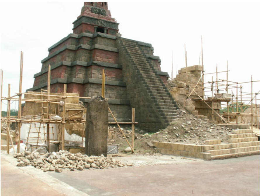
Fig. 8.21 The damaged and weathered structure in the Central Plaza of the Apocalypso cityscape undergoing remodeling and construction with more Postclassic architecture forms burying the Classic period building (Photo: R.D. Hansen)
